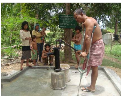
Drilled Well for Disabled family in Prek Toch commune, Maung district provided by AAM
